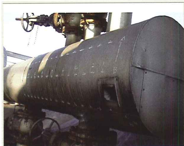
Fig 9: Monitoring heat exchanger shells.
